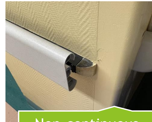
Non-continuous handrail / sharp
